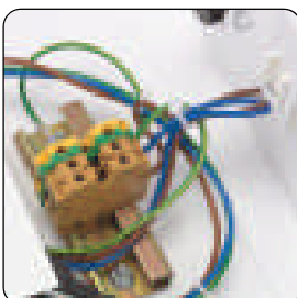
Terminal block access
