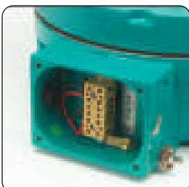
Terminal Block Access
