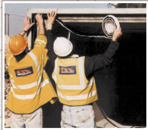
Tokstrip is applied to the primed joint of a box culvert unit.
