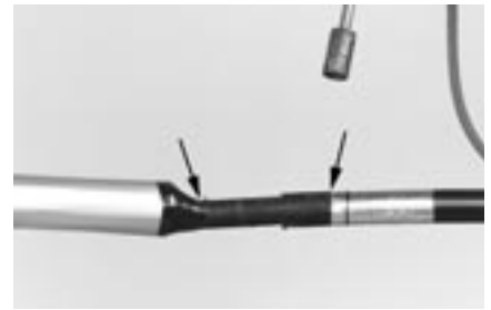
15 Flame brush the cable areas with a soft flame for about 10 seconds, as indicated between the arrows.
