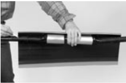
13 Centre the sleeve over the splice and mark the ends on the outer cable jacket.
