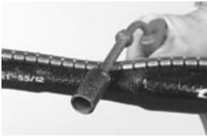
19 When all the green paint has turned to black on the the first half of the closure, support it and press down the channel with a suitable tool following the transition from the liner/sleeve area.
