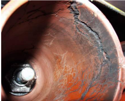
Figure 1 – Damage caused by surface PD activity
