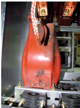
Figure 2 – Treeing surface erosion on a current transformer
