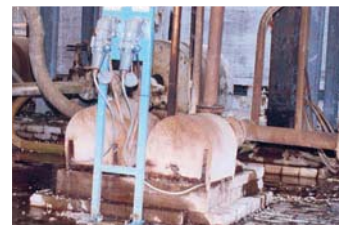
Pumps in wet atmosphere
