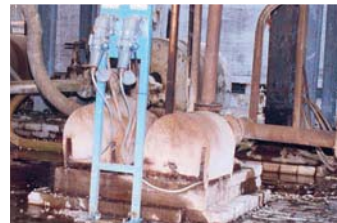
Pumps in wet atmosphere
