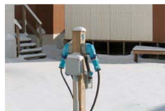
External power supply for water treatment
