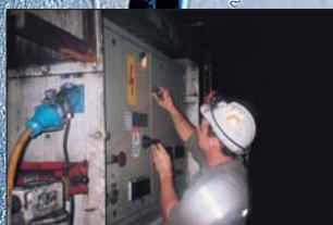
Power supply to generators
