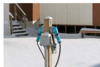
External power supply for water treatment
