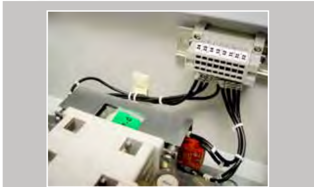
Interior view showing flag indicator and the auxiliary blocks wired down to terminals.
