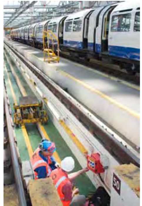
Application in Rolling Stock Repair pits
