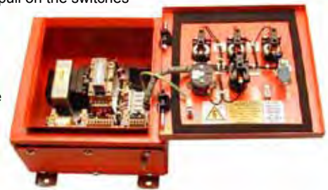
CS1 Control Station Interior
