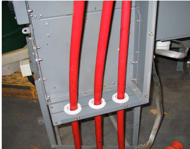
Completed installation (termination or earthing not shown)
