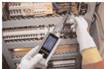
Control over board with M-952271
