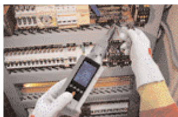
Control over board with M-952271
