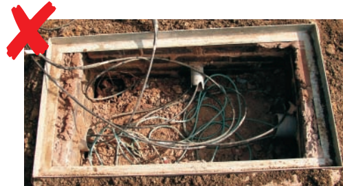
Unacceptable standard of finished box
