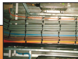
Marine Cable Bundling
