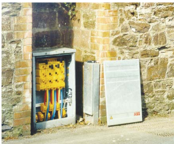
Junction box installed in Bristol, England.
