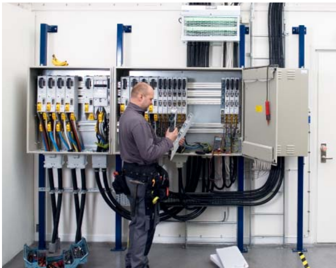
Cable distribution board in powder coated enclosure mounted on the wall at the bakery shop in Gothenburg, Sweden.
