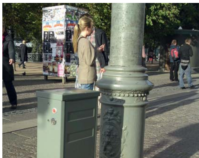
Cable distribution cabinet, Brunnsparken, Gothenburg, Sweden.
