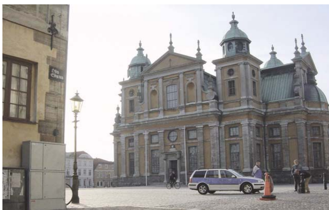
Cable distribution board used for streetlighting near Kalmar cathedral, Sweden.
