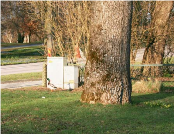
Cable distribution cabinet in a in Alingsås, Sweden.
