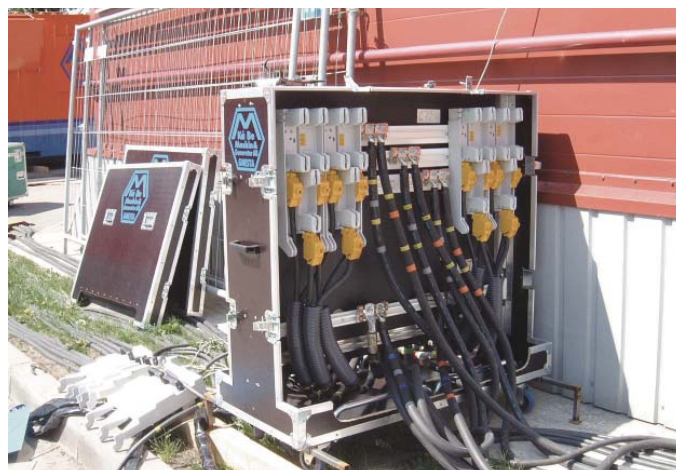
Temporary service distribution boards for the "Eurovision Song Contest 2003" in Riga, Latvia.
