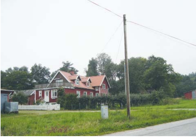
Cable distribution cabinet, Säby, Sweden.
