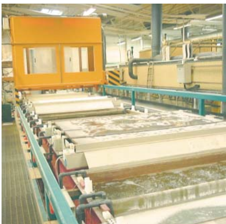
Automatic hot-dip galvanizing plant.
