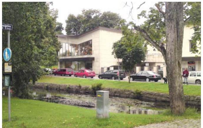
Kabeldon cable distribution cabinet nearby Alingsås library, Sweden.
