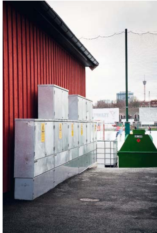
Cable distribution boards at Hedens bandy rink, Gothenburg, Sweden.
