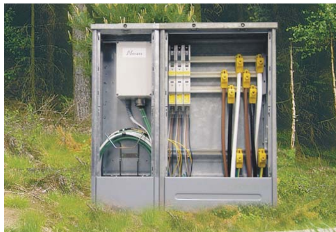
Cable distribution cabinets used for electricity and fibre optic networks.
