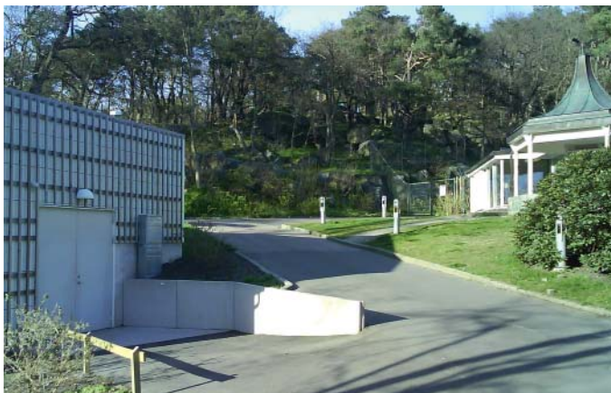
Cable distribution board in Slottsskogen, Gothenburg, Sweden.
