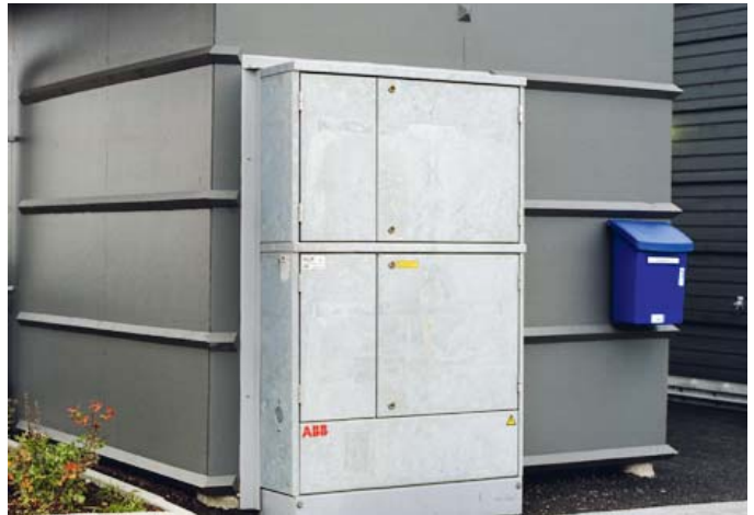
Cable distribution board, Mc Donald's, Sweden
