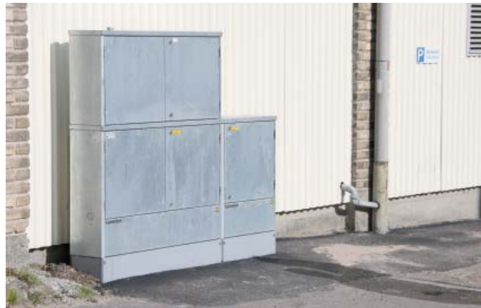
Cable distribution board in Malmö, Sweden.
