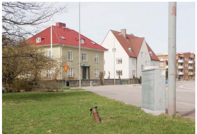
Cable distribution cabinet in Varberg's housing area, Sweden.
