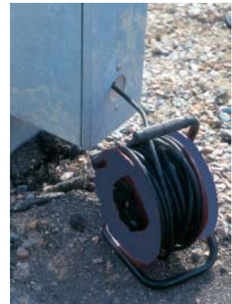
The openings on the sides of the cabinet is used for temporary power outlets, etc.
