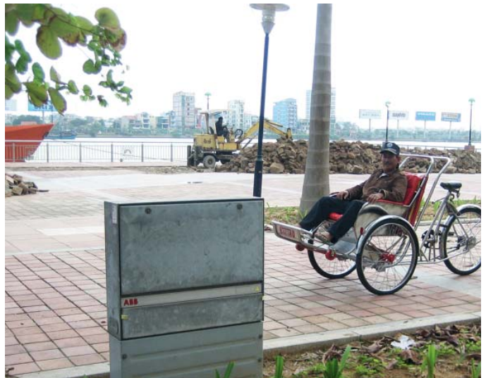
Kabeldon cable distribution cabinet, Vietnam.
