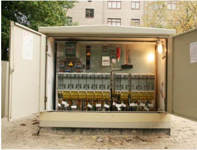
Kabeldon switching devices in substation distribution, Latvia.
