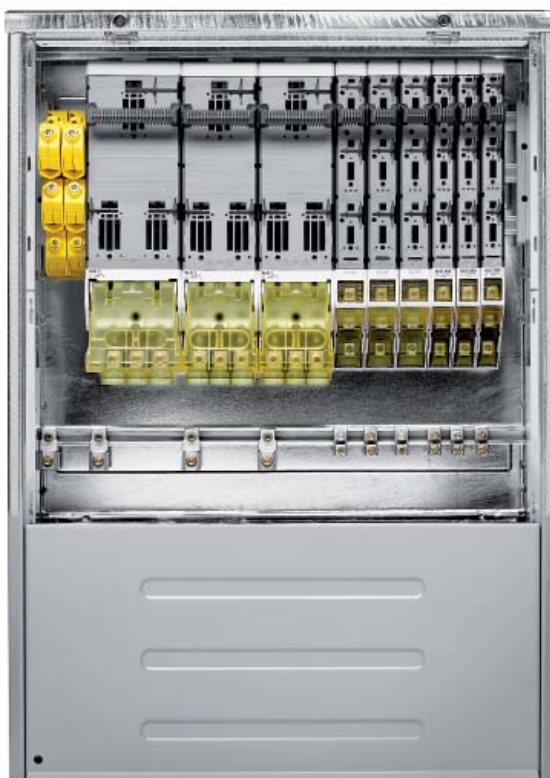
Cable distribution cabinets with switching devices and busbar systems.
