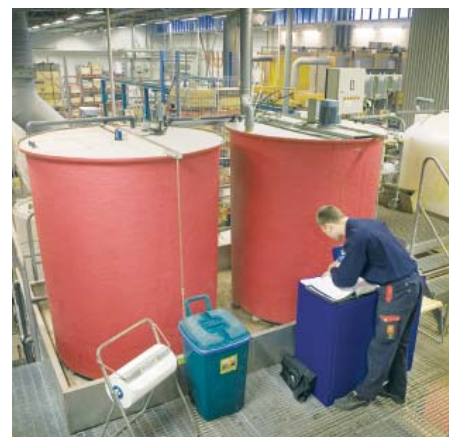
Treatment for outgoing waste water from surface treatment.
