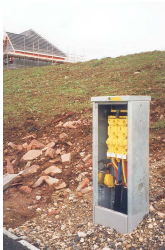
Junction box installed in Bristol, England. This replaces the conventional underground junction box.
