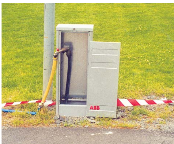
In Jönköping, Sweden, a CDC enclosure has been used for the water supply for the trade fair site.
