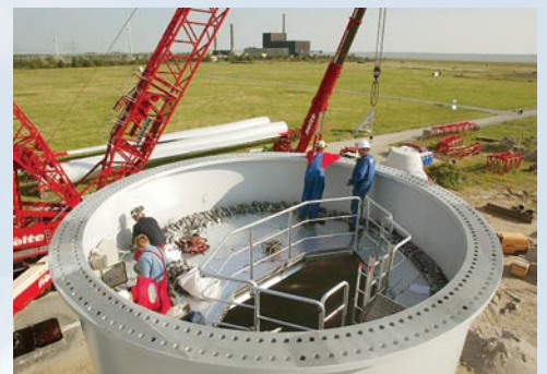
Proper grounding of the tower during construction is essential for preparing the wind turbine for lightning strikes.
