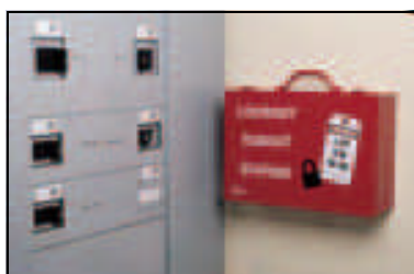
Mount close to power and distribution panels
