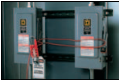
Lockout Single or Multiple Disconnects
