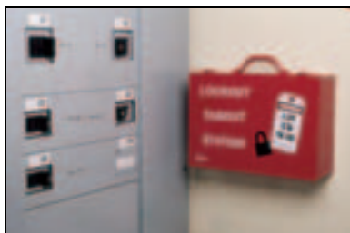
Mount close to power and distribution panels
