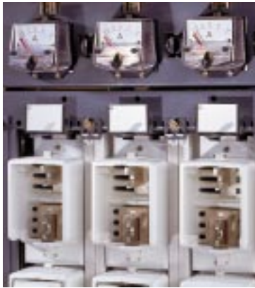
Load monitoring of outgoing circuits
