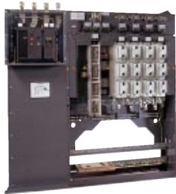
Fuseboards with incoming circuit breaker and outgoing fuseways.
