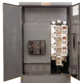
Flexible supply for larger ratings, combine ACB and Shielded fuseways within a Feeder Pillar.
