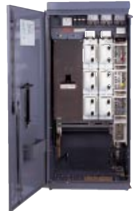
Fuse cabinet with 2 x 630A Shielded fuseways and up to 1250A outgoing MCCB.
