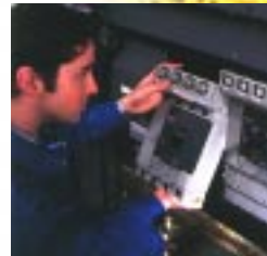
Adding additional circuits
