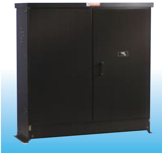
Stainless steel clad package substation for Hong Kong.
