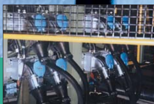
Power supply to production lines
