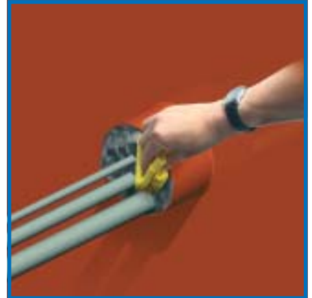
With a damp cloth the FIWA® sealant is forced into and between the empty sleeves to ensure a homogeneous filling.
