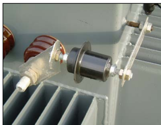
Neutral Point LV Surge Arrester
