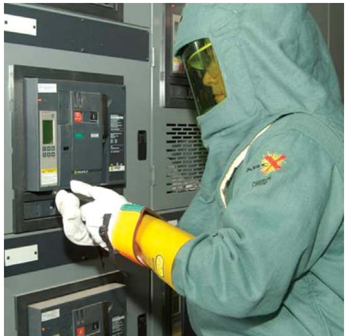
Personal protection equipment for defence from arc flash
