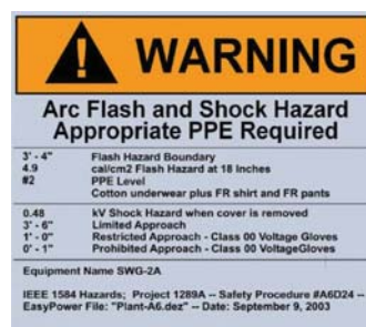
A typical ARC Flash warning label
