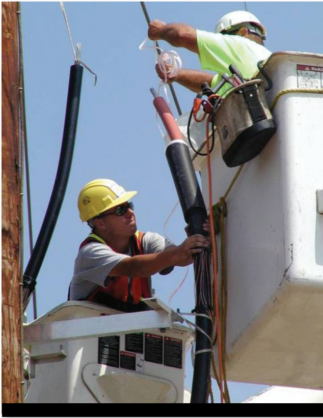
Steve Norvell holds the semiconductive cold-shrink tube as the core is removed.
